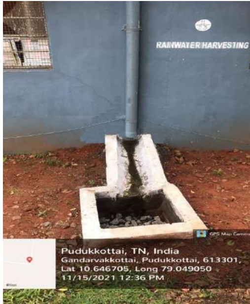
Rainwater Harvesting system at Block IV
