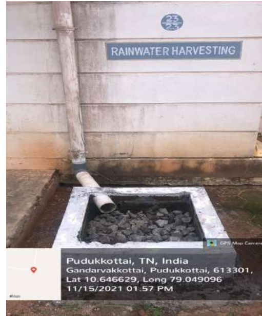
Rainwater Harvesting system at Library
