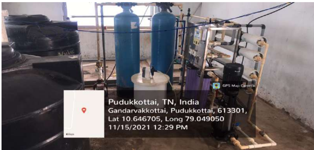
Reverse Osmosis Plant (RO)
