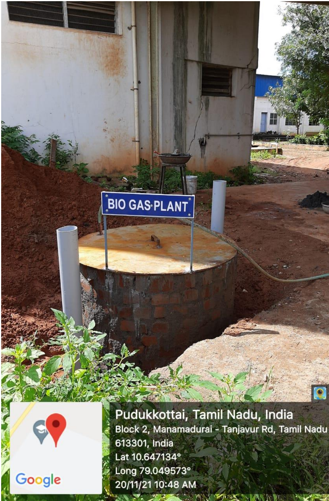
BIO GAS PLANT
