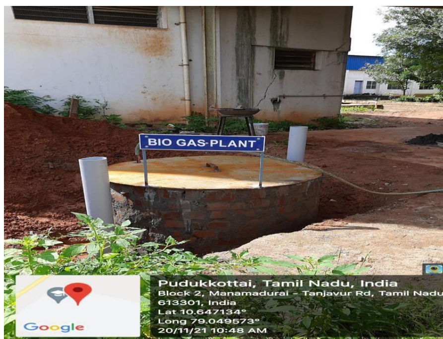
Photograph of Installed Mini Bio Gas Plant
